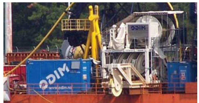
The fibre rope deployment system assisted installation in water depths of 2731 m
