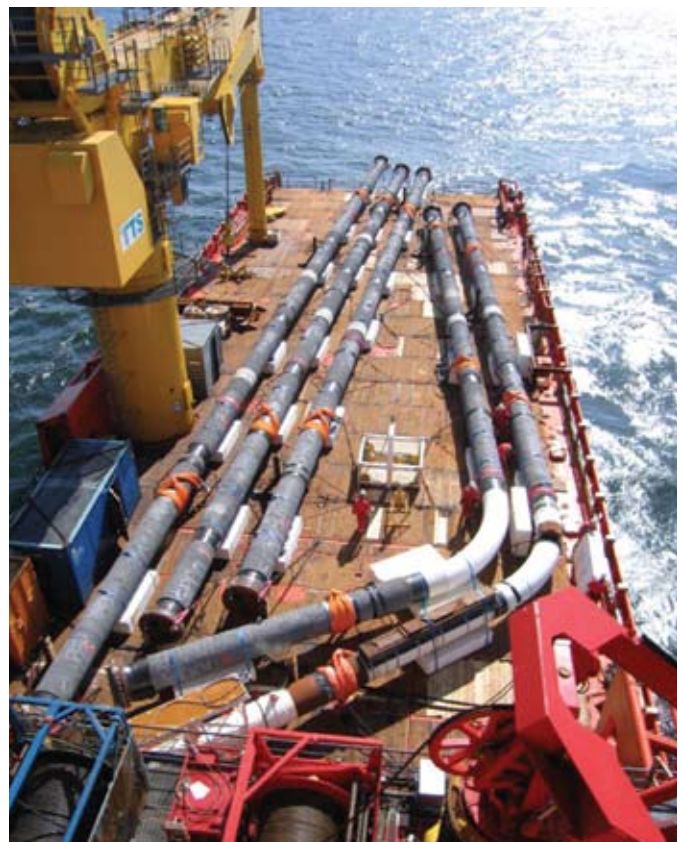
Spool pieces were transported and wet stored using the Edda Fjord, Multipurpose Platform Supply Vessel
